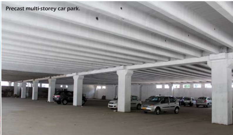
SRM University is constructing an 11-storey hostel building at Trichy in Tamil Nadu, accommodating a large column-free space at ground floor. To achieve the column-free area, innovative use of precast moment frames is adopted. The flooring is in the form of precast, pre-stressed hollowcore units.
